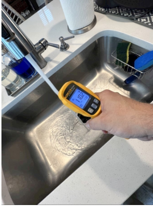
Water Heater: Average temperature at fixtures was 110° F.
