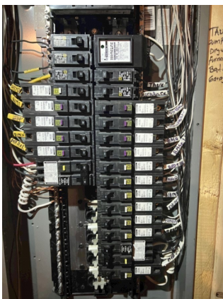
Electrical: Branch circuits also labeled inside panel
