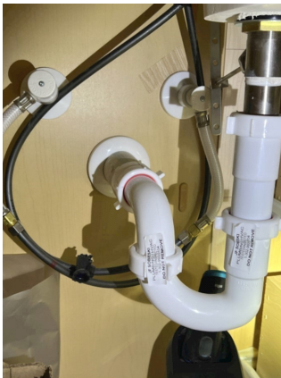
Plumbing: All fixtures have shut offs located near the fixture
