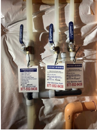
Plumbing: Main house, front and rear hose bib shut offs
