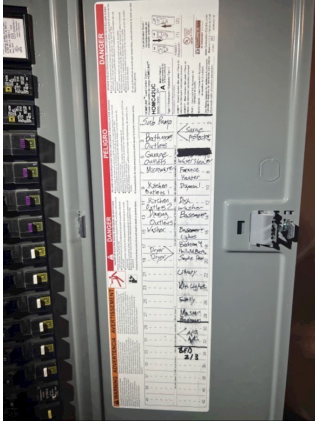
Electrical: All circuits properly labeled inside panel door
