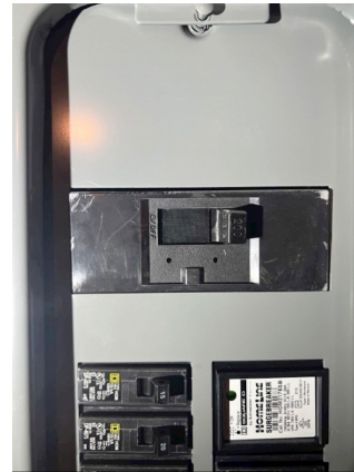
Electrical: Service main cut off breaker
