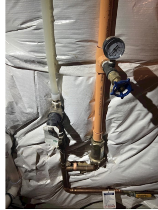
Plumbing: Water service main and sprinkler system drain valve
